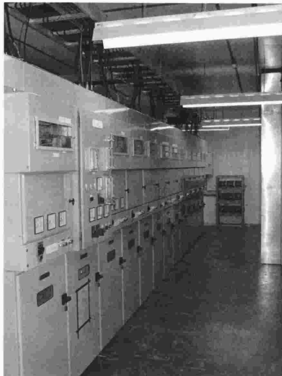
Half of the switchboard.
