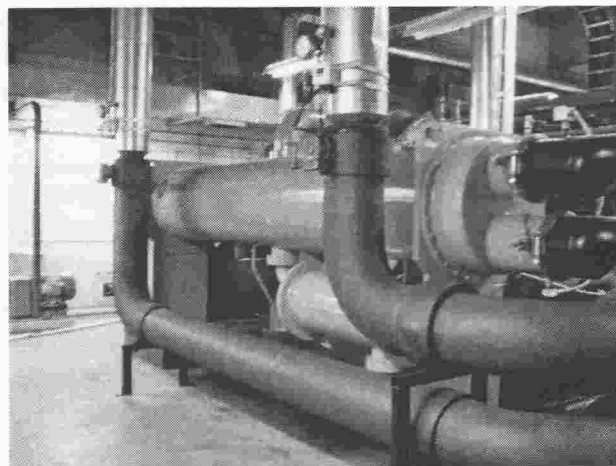
One of the older chiller units
